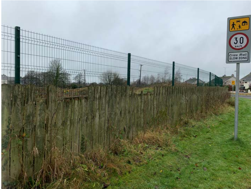
Plate 2-12: Damaged Fencing at Coille Dios
