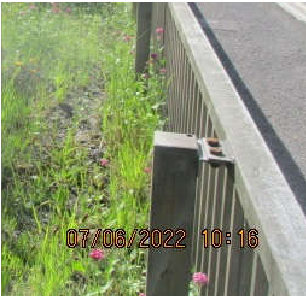
Plate 4.2 - Made ground on east side of railings with grass encroachment.
