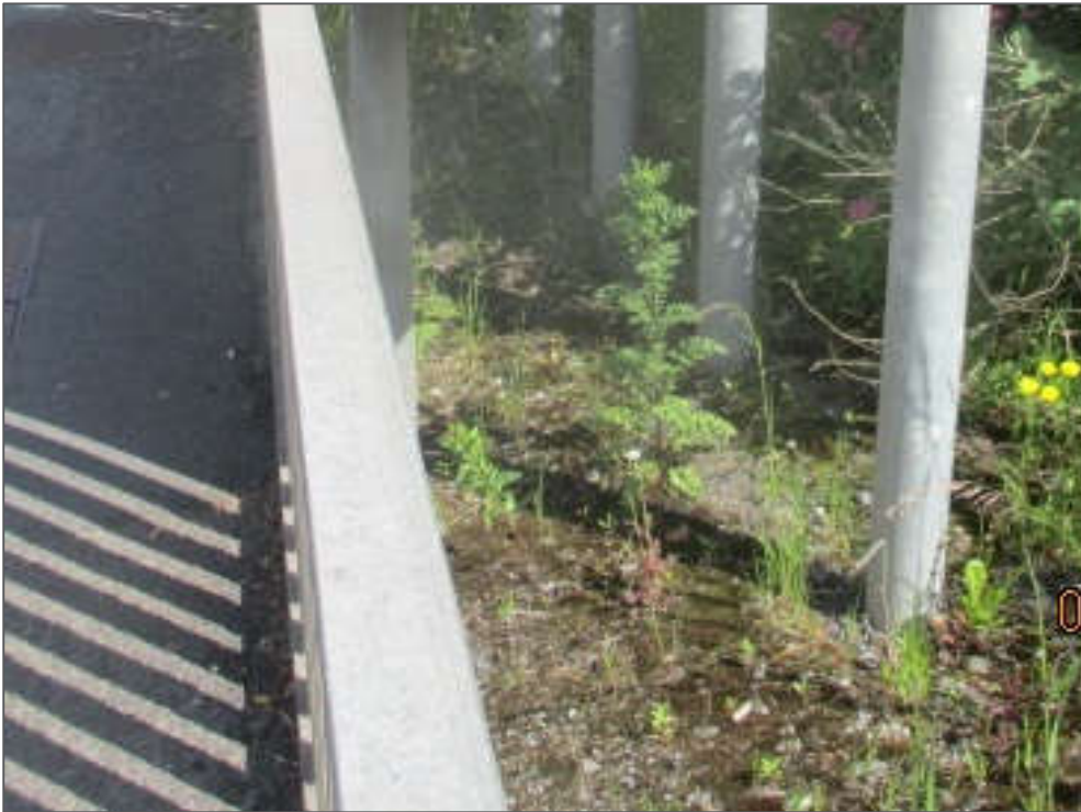
Plate 4.1 - Made ground on east side of railings
