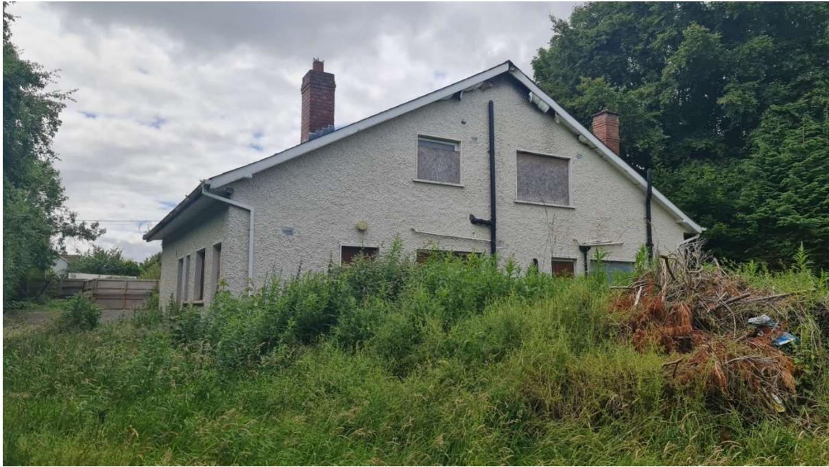
Rear elevation, with significant overgrowth in the foreground.
