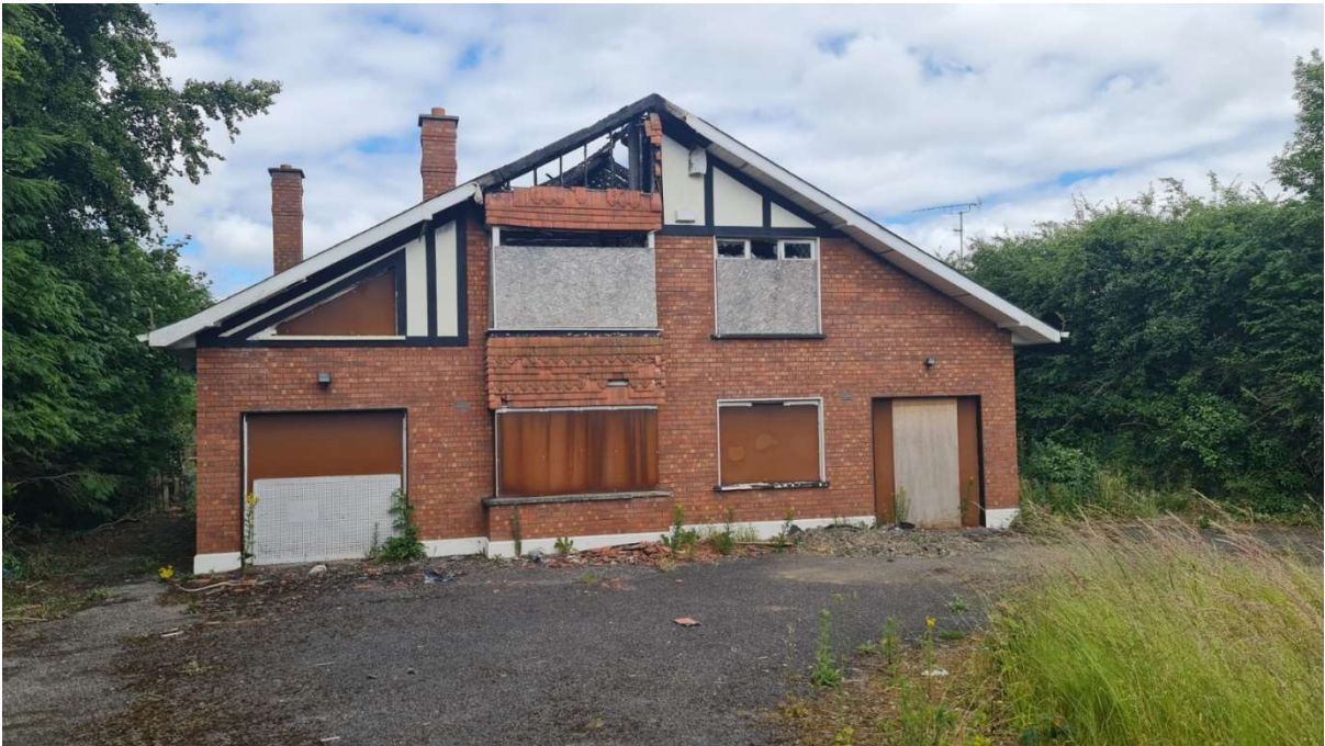
Front elevation of property with partially collapsed roof and wall at high level
