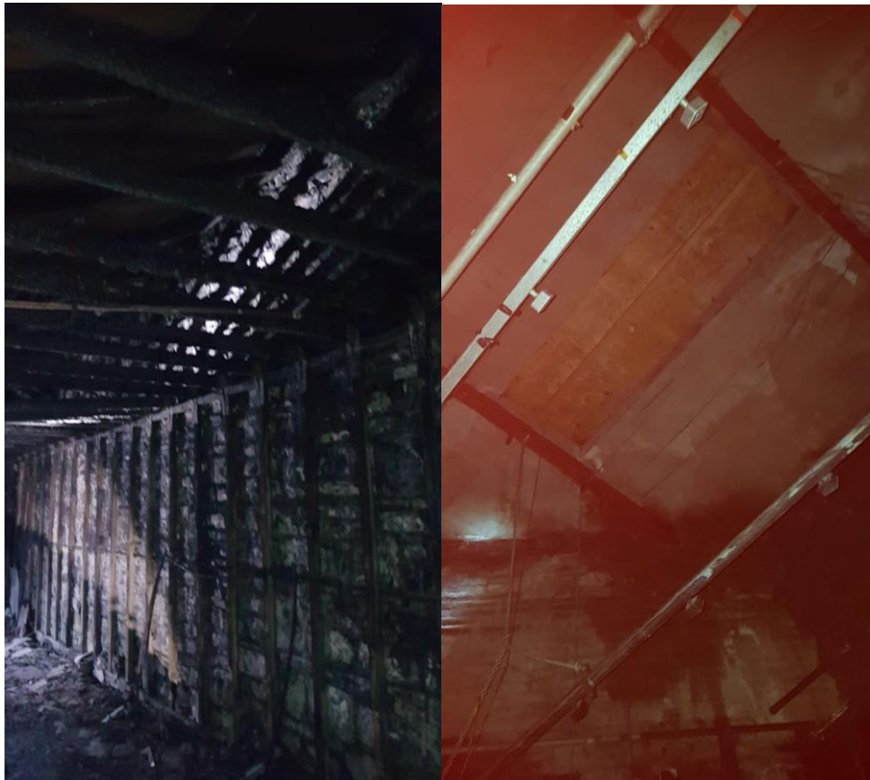
View of attics and spaces within the Market House, Bingo hall and small shed (burnt out)
