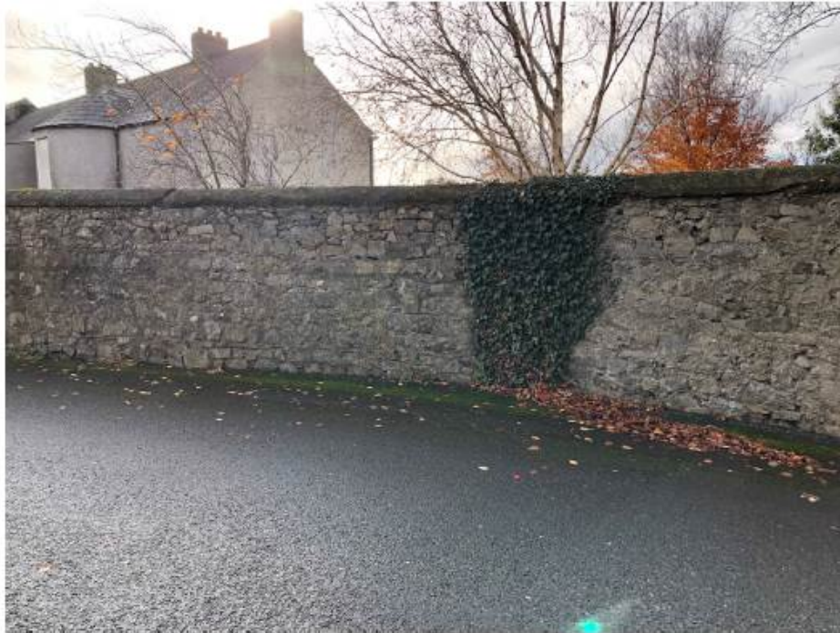
Detail of gap in wall close to castle, the end of proposed wall realignment on the north side of the road.
