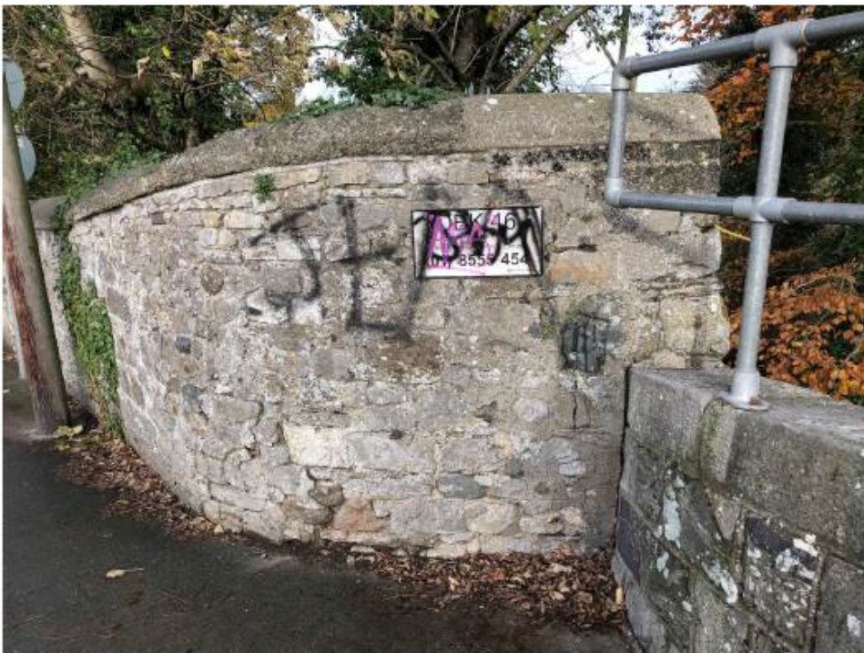
Detail view of end Loreto Convent wall at bridge showing damage, repairs and range of techniques, curved section is built on top of 1850 bridge. Note crude guarding to be replaced.
