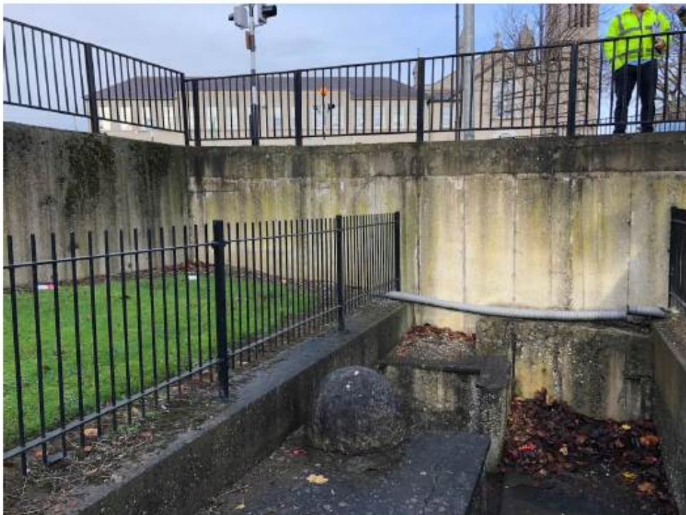
View from level of well looking towards existing retaining wall along Circular Road.
