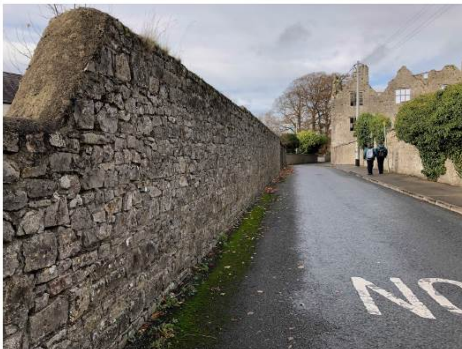
Detail of wall section from junction with Elm Road showing coursed rubble in bands, suggesting a later construction date to the wall section closer to the castle.
