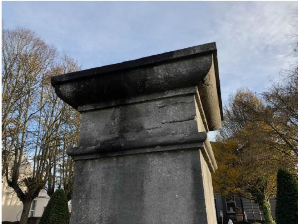
Detail of decayed stone to gate pier.
