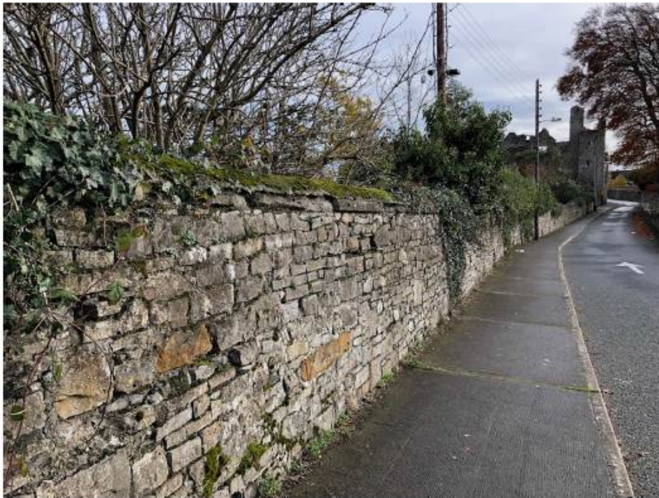
View looking east along road towards Athumeny Castle, showing coursed faced rubble, parallel to road incline with domed lime capping and damage, likely due to historic ivy coverage.
