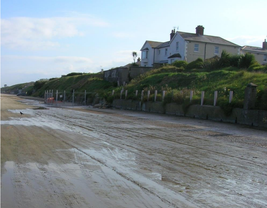
Photograph 7.4: View looking south showing collapse of sea wall (note wet sand conditions)
