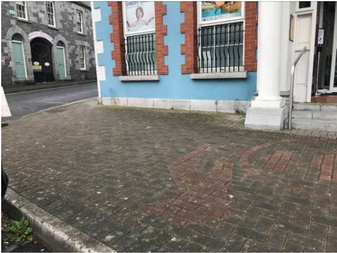
The diminishing depth of the plinth on the southern side of the building illustrates the issue with falls in and around the building.
