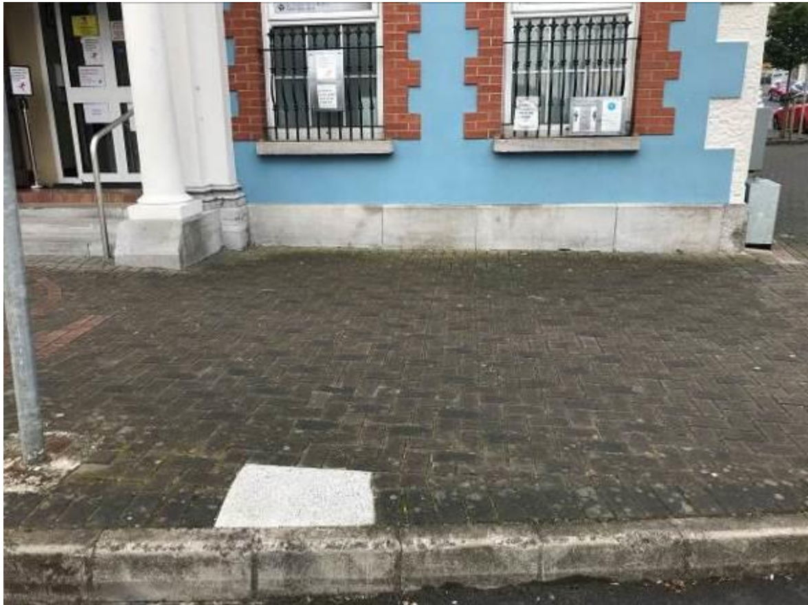
Ground floor at junction with paved forecourt. The brick reveals are not original and detract from the appearance of the building. The stone plinth is an important element of the composition and needs to be retained as a feature of the elevation. A purely functional design response to the need for a ramp could negatively impact on the plinth and take away from the setting and proportions of the front elevation.
