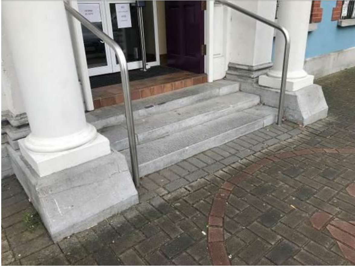
The lack of universal access and the challenges for people with prams are clear to be seen at the front entrance. As part of the public realm works, this will be resolved.
