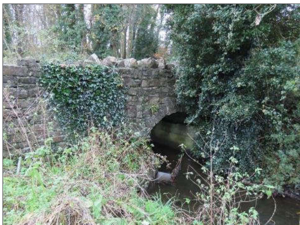
Plate 4.26 Bridge 2 (James Corbally Bridge) – upstream elevation – single masonry arch with concrete abutments.
