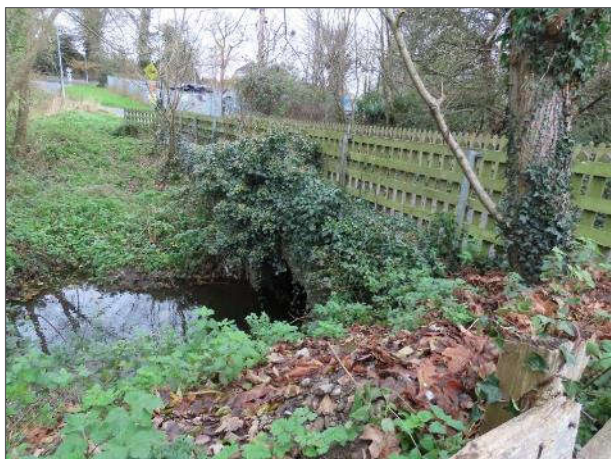
Plate 4.38 Bridge 3 – upstream elevation – heavily overgrown with ivy.
