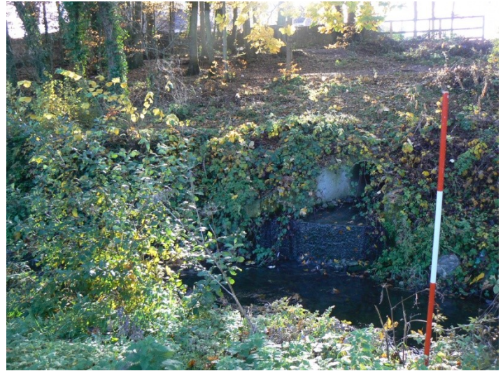
814D. E End. Facing E with 814F with culvert to rear. P1200430
