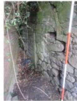
IMG_0096 'Smithy' blocked W wall
