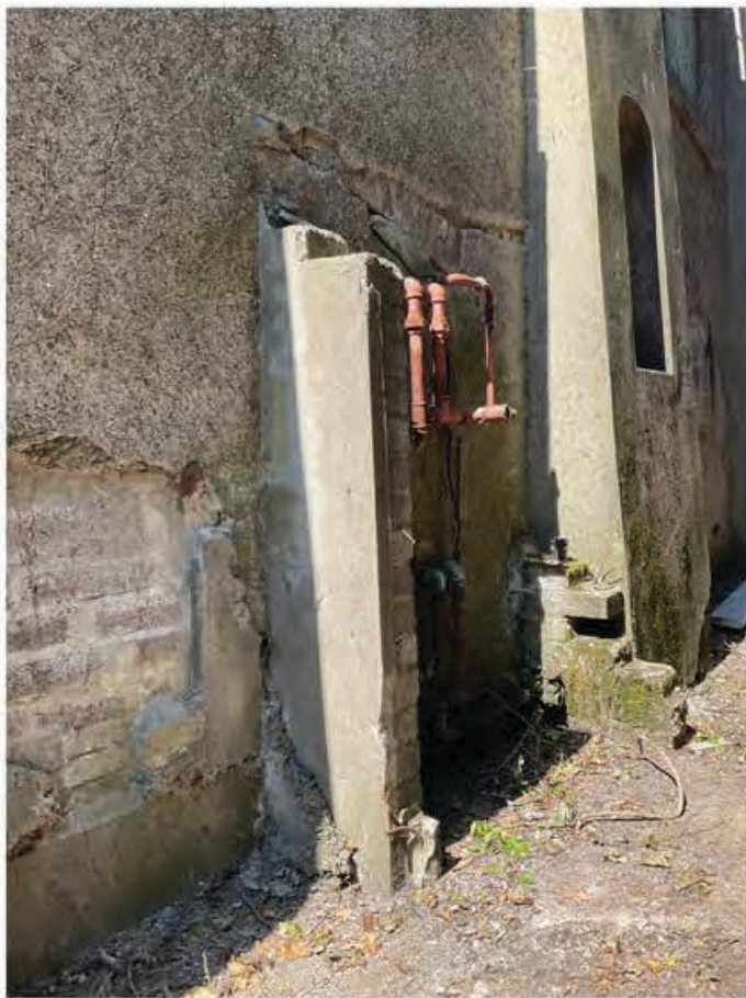
2.9 Disconnected services - East wall.jpg
