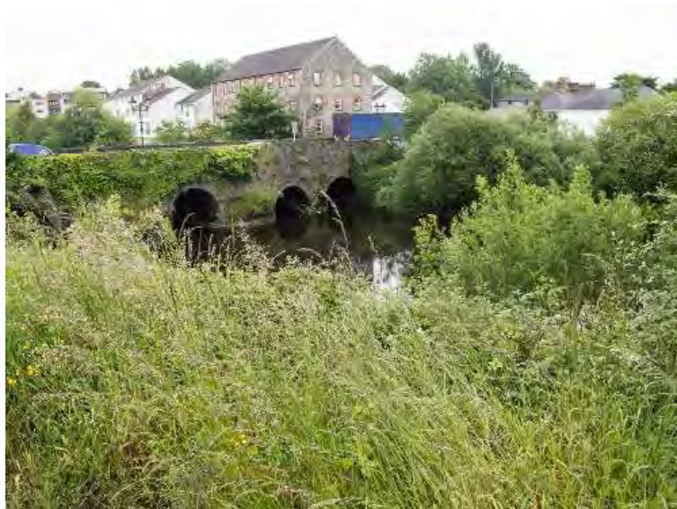
Figure 6: South-facing aspect of the bridge. Removal of the (mostly) ivy will enhance lichen growth provided the structure is not chemically cleaned.
