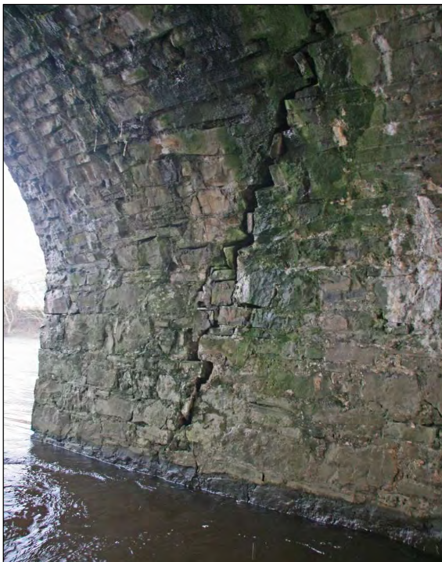
Plate 13: Crack in third arch from western side of bridge
