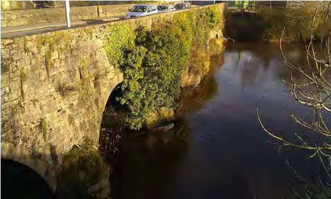
Figure 6: New Bridge with old stone walls (BL1), ivy and other species are found here. The pedestrian bridge is proposed for this south facing side of the bridge. The bridge was cleaned after this photograph was taken in 2013 and as at March 2016 there was no ivy present.
