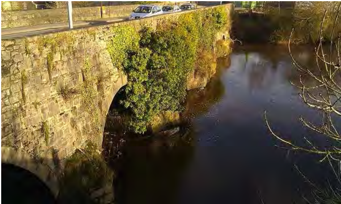
Plate 1: New Bridge with old stone walls (upstream view). The pedestrian bridge is proposed for this south facing side of the bridge (photo taken in 2013 prior to ivy removal and bridge cleaning in 2015).
