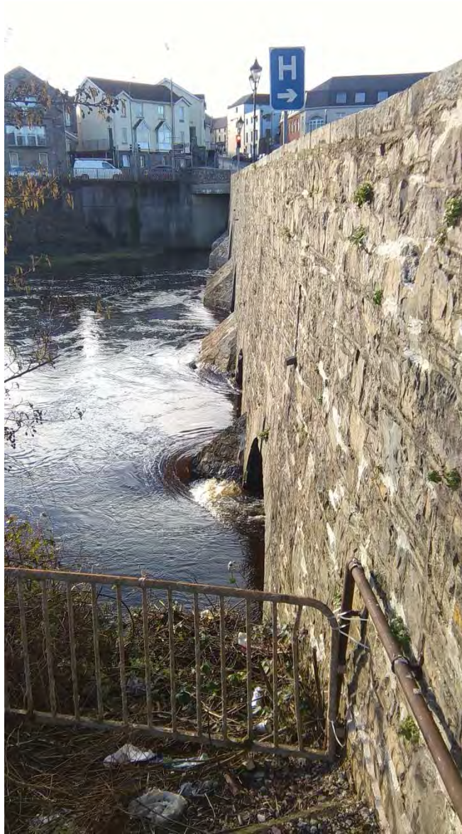
Plate 2: New Bridge upstream, view from the bank opposite to that in Plate 1, above. Photo taken in February 2016, after cleaning works had taken place in 2015).
