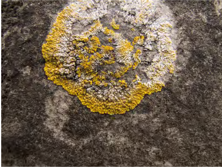
Figure 2: Few and poorly developed Caloplaca flavescens on the vertical aspect of the bridge walls. Normally a lot more of this species would be expected.
