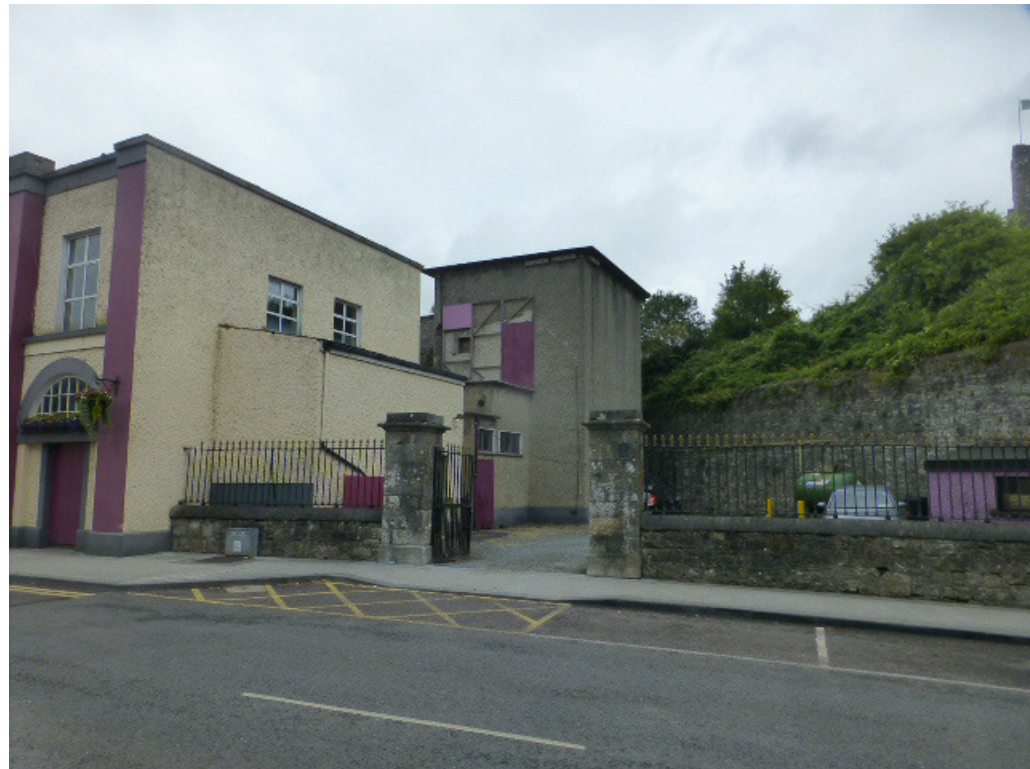
Fig 21. South gable facade with lean-to structure and 1950's fly-tower of ballroom to rear .
