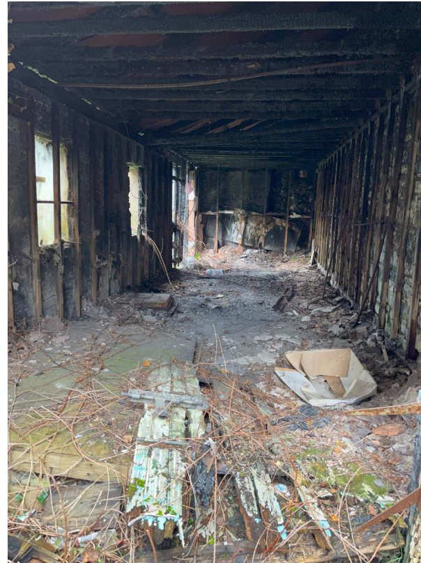
Fig 32. Interior view of lean-to structure - building in poor condition due to extensive fire damage.
