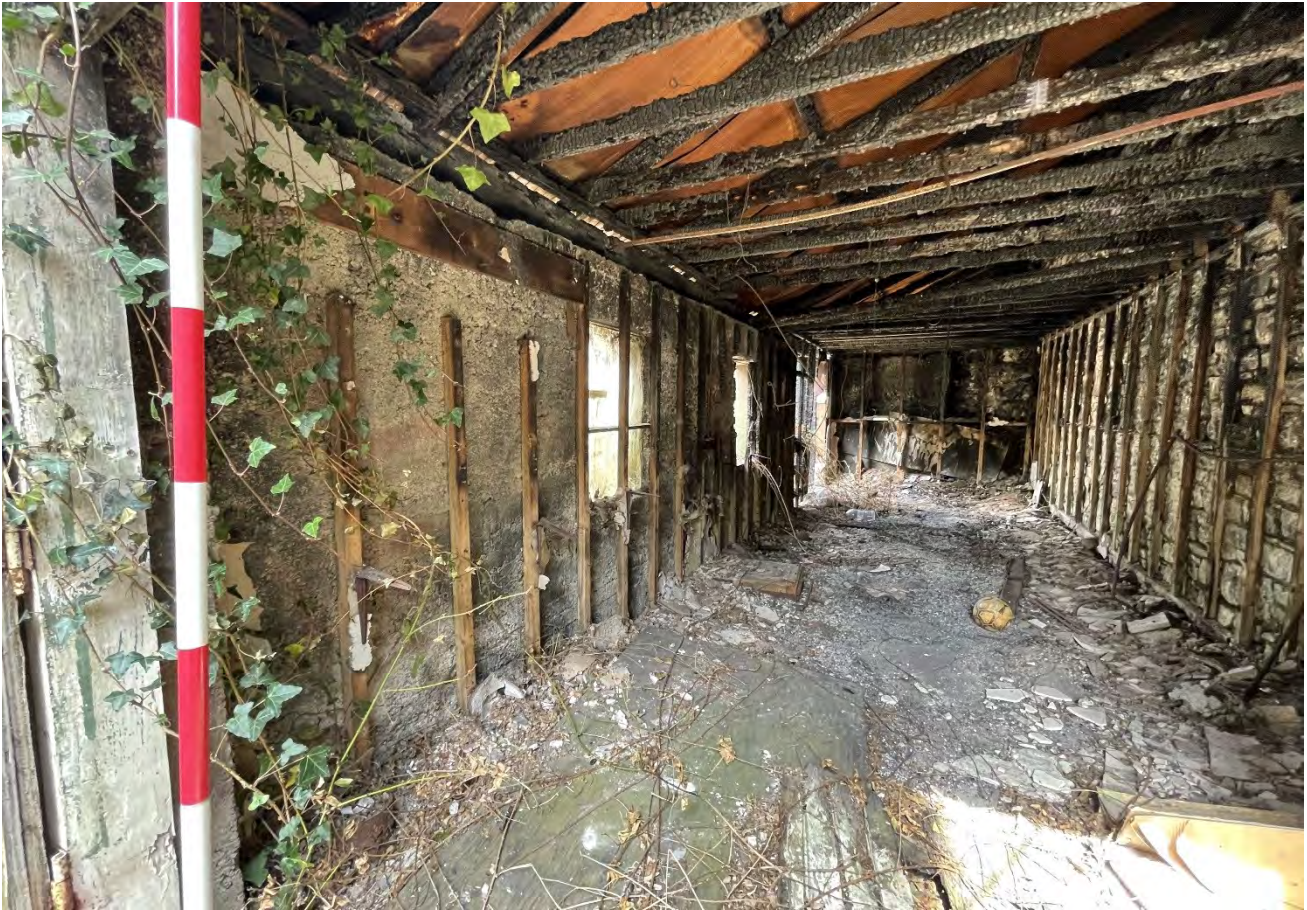
Plate 15: Burnt interior of the lean to shed, facing northeast.
