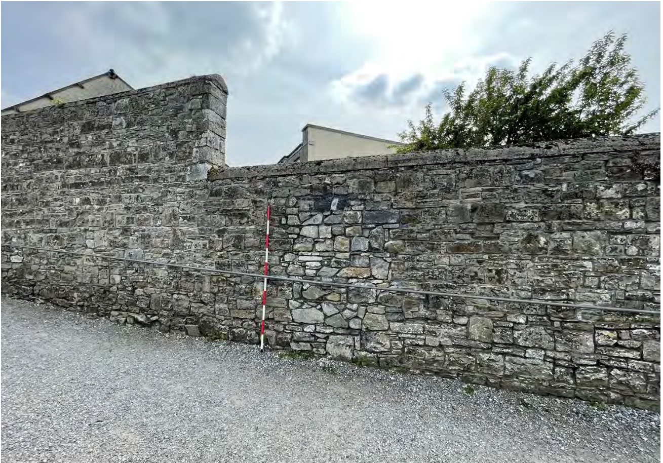
Plate 29: Detail; repair visible in the north façade of the south wall flanking the causeway, facing south.
