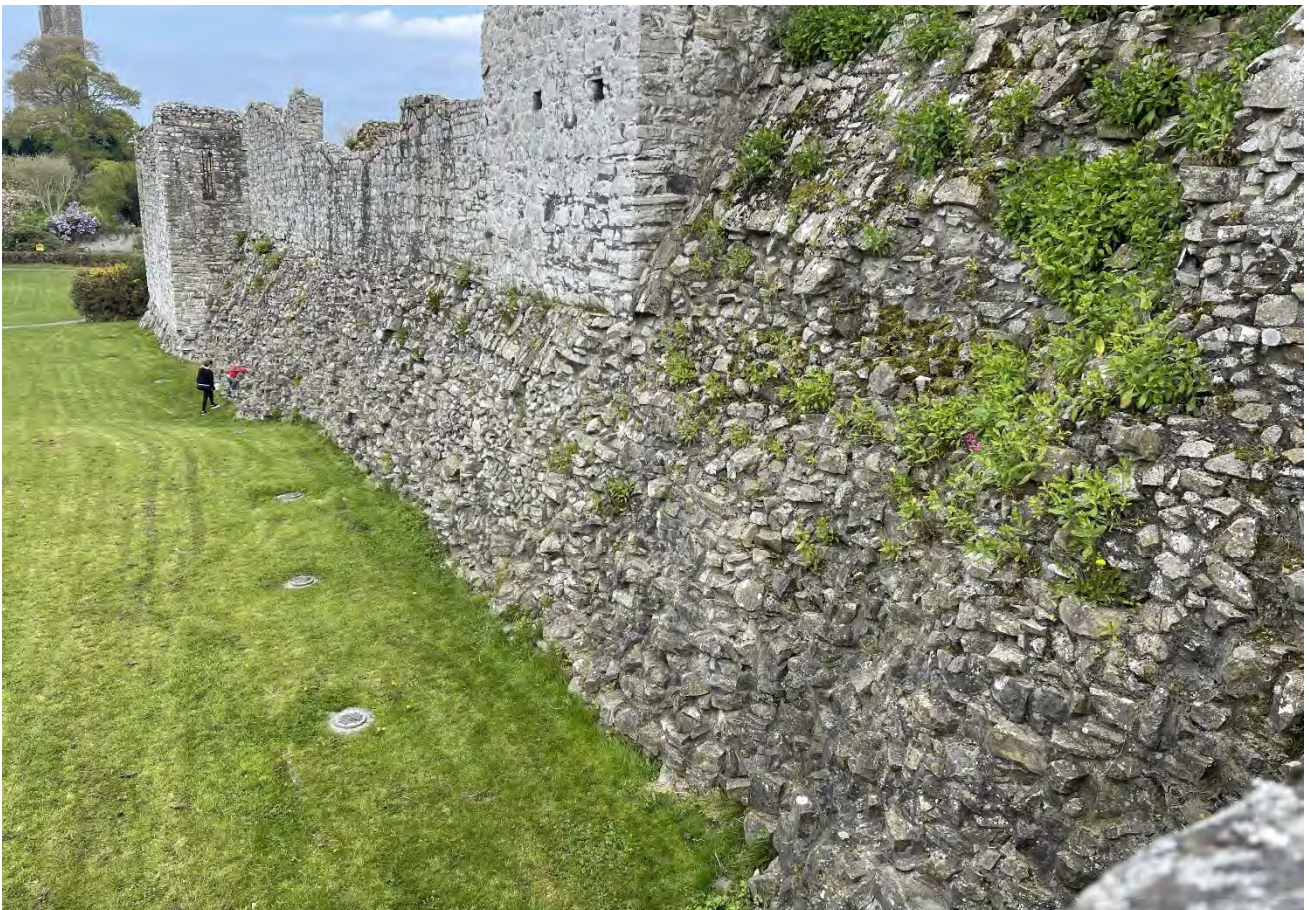
Plate 42: Northwest facing façade of the curtain wall with sloping, external base batter visible, to the north of Trim Gate, facing northeast.
