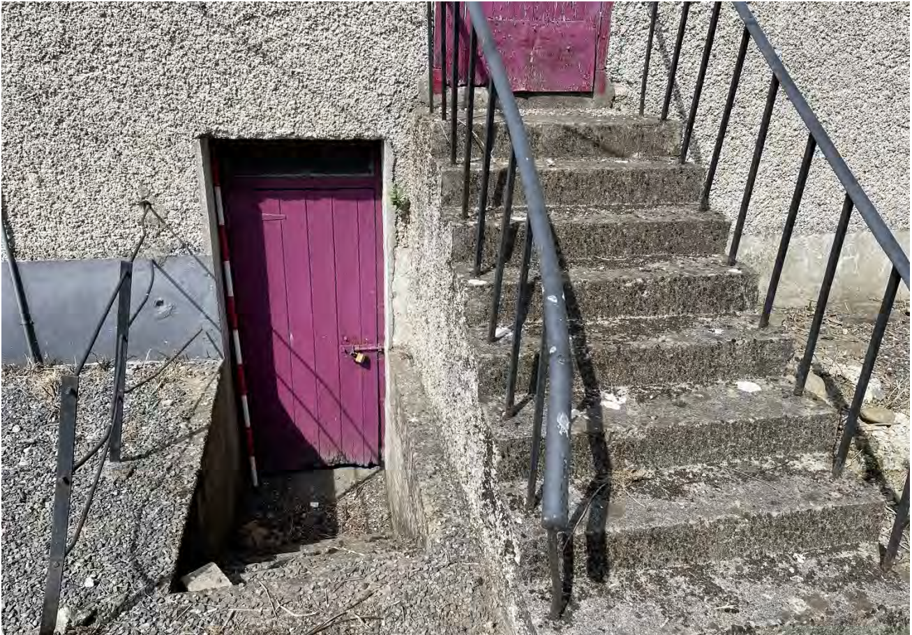
Plate 11: Access to the under-stage area of the fly-tower of the ballroom, facing north.
