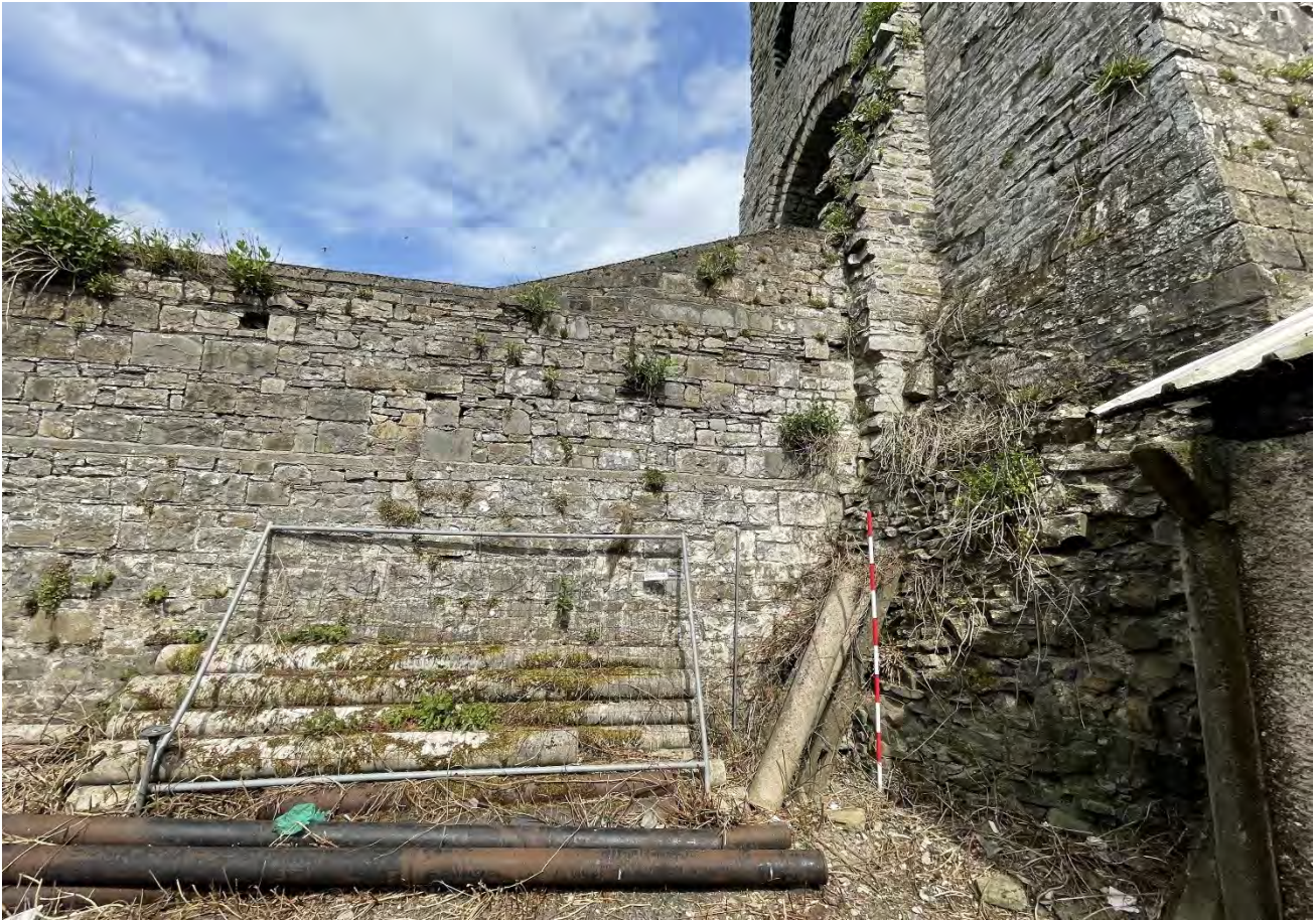
Plate 19: South façade of the causeway wall, external base batter/glacis of Trim Gate visible, facing northeast.
