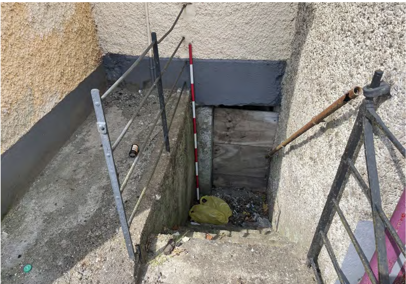
Plate 12: Access to a basement area below south-east corner of 1925 southern additional bay of Market House, facing north.
