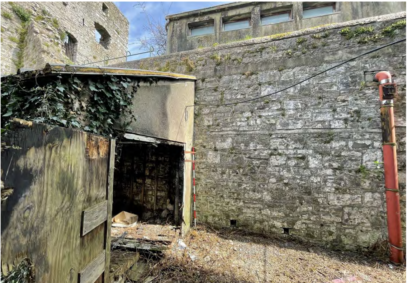
Plate 16: Detail, lean to shed built against the 19th century modern wall. Sewer pipe visible, of toilet building above within the keep, facing south.
