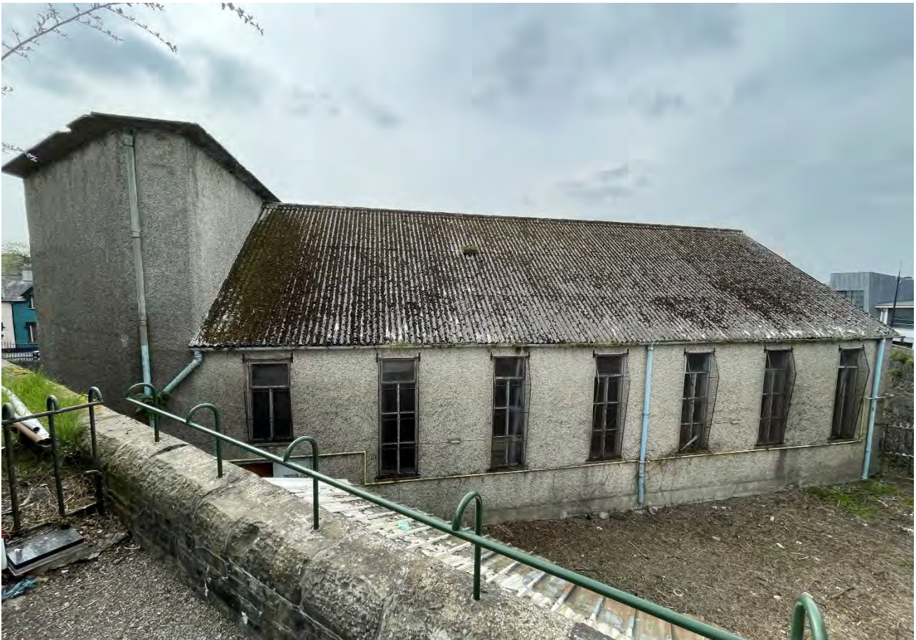
Plate 35: View of the rear of the site and the east elevation of Ballroom, facing west.
