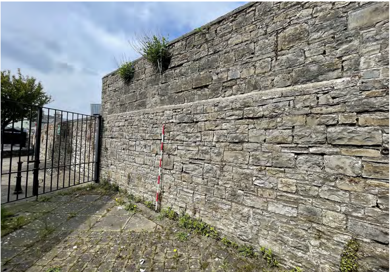
Plate 26: South façade of causeway wall, rear of the site, facing southeast where proposed walkway will penetrate wall
