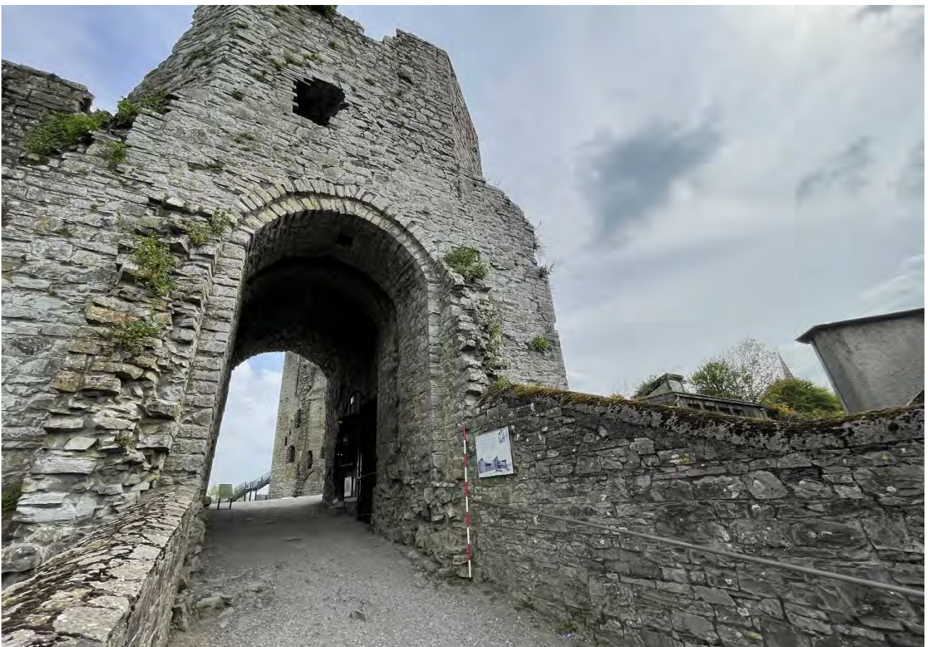
Plate 30: Trim Gate, with stub remains of original flanking walls visible, facing southeast.
