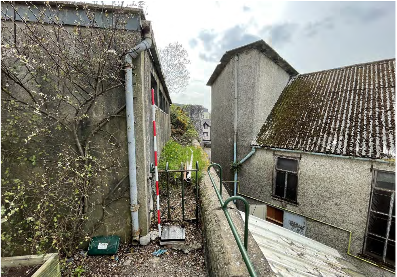
Plate 37: Toilet building within keep, built on the top of curtain wall footprint, facing southwest.
