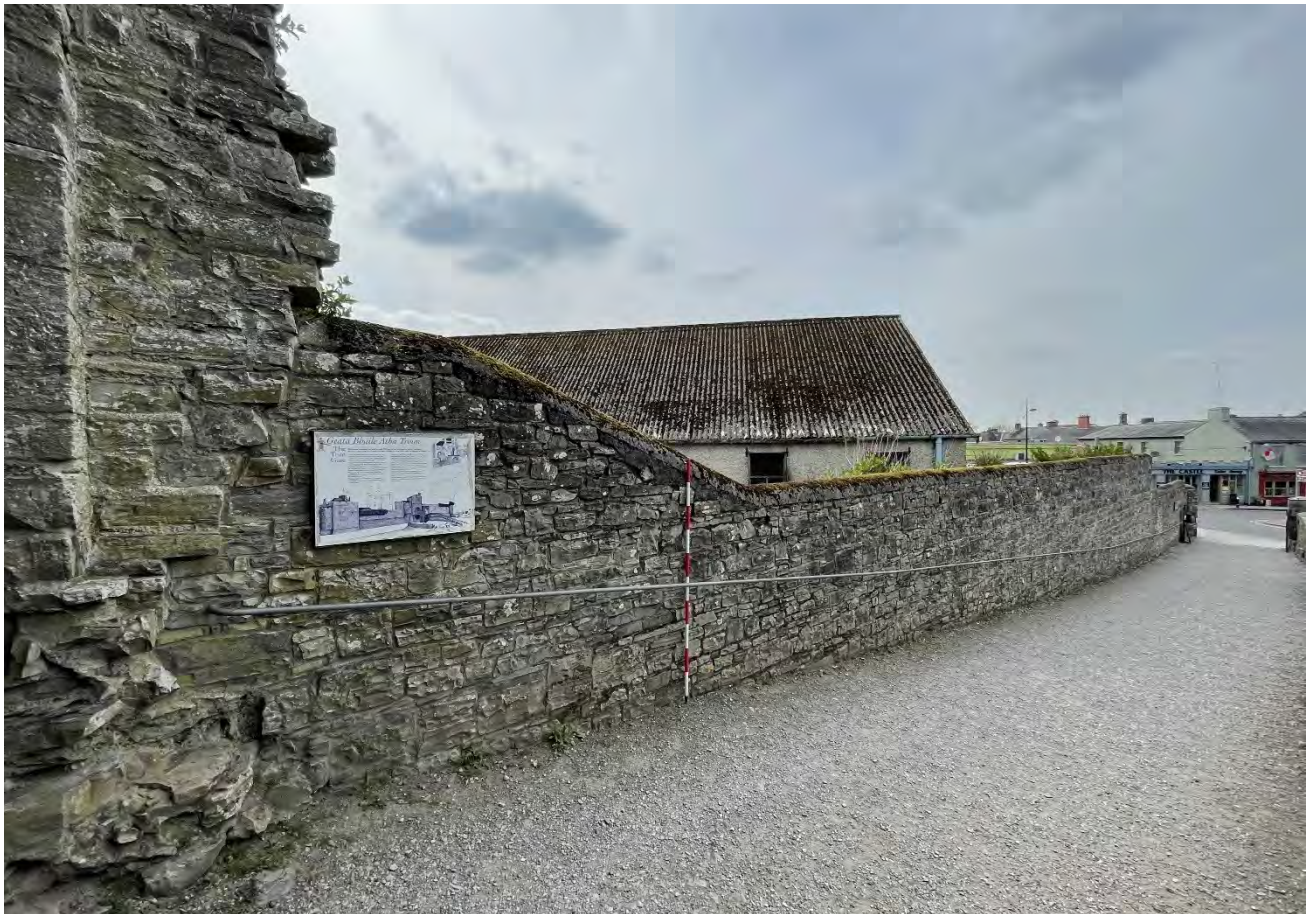
Plate 31: View of the north façade of the existing south flanking wall, facing west.
