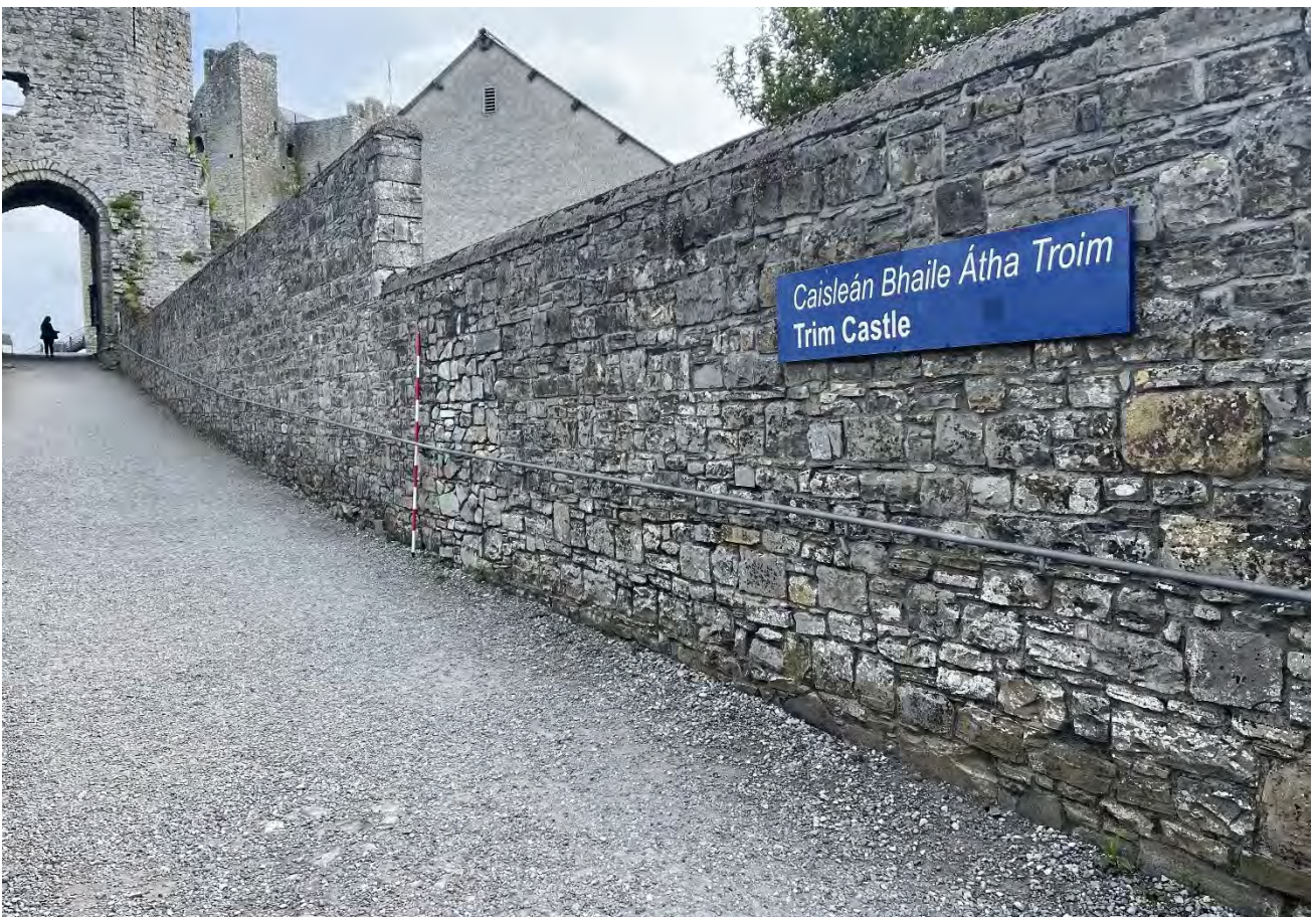
Plate 28: North façade of the south wall flanking the causeway, facing southeast. Proposed walkway will penetrate at location of range rod approximately
