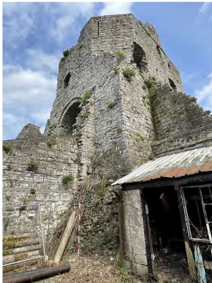
Plate 18: Detail; Trim Gate, with rough base of the foundation batter of tower visible, facing east.
