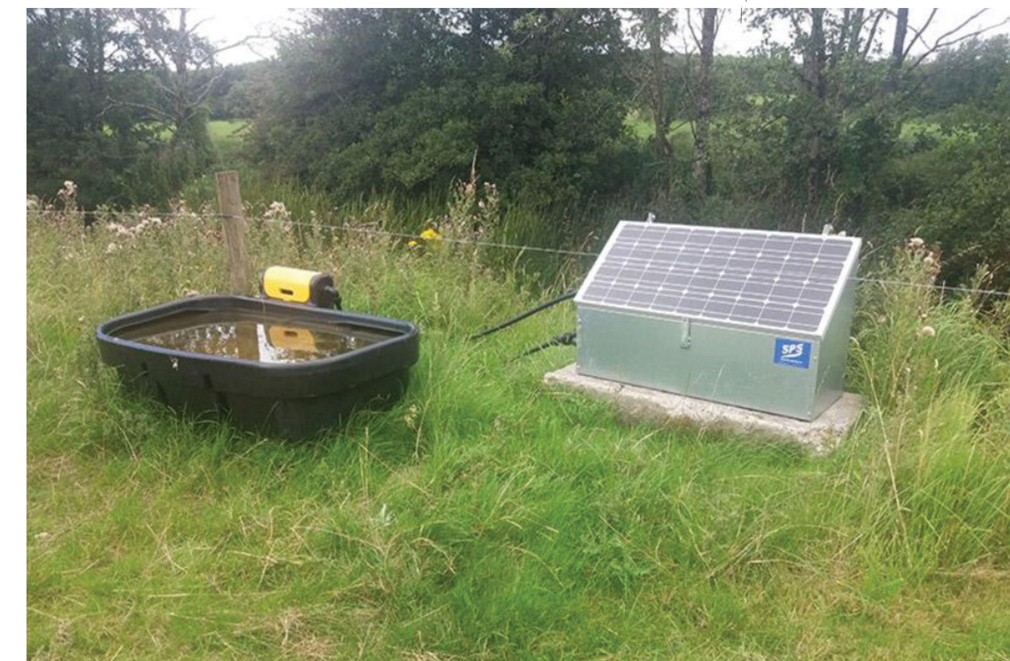
Drinking troughs to be placed at movable sites at least 20m from shore. The use of solar powered pumps allow water to be brought up the slope to troughs at various locations.
